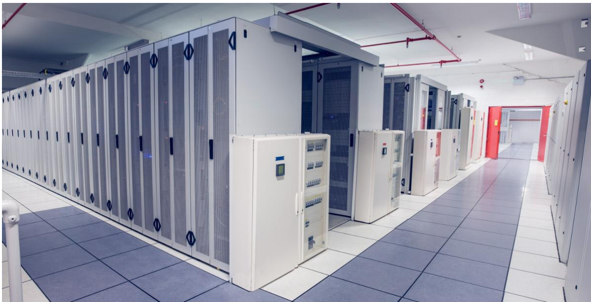
Figure 2 Internal Data Centre
