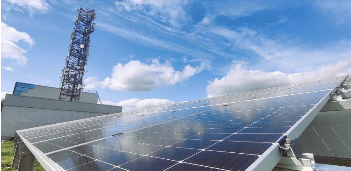
Figure 8 Solar PV System
